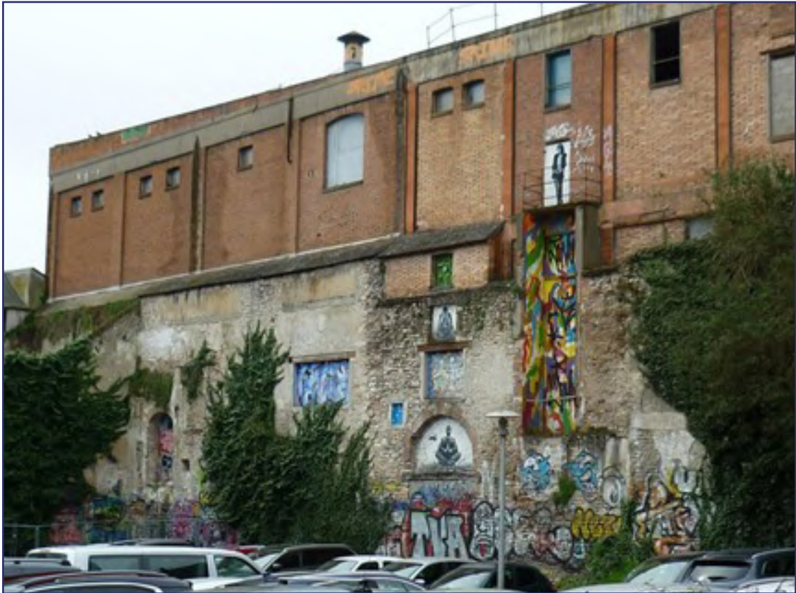
Fig. 2.2.3.4 The Dessaux Vinegar Factory, a brownfield located in downtown Orléans. (Source: Personal archive, 2025)
