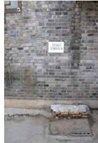
Figure 4. The covered catch basin and the warning sign on the wall (Source: author photo)
