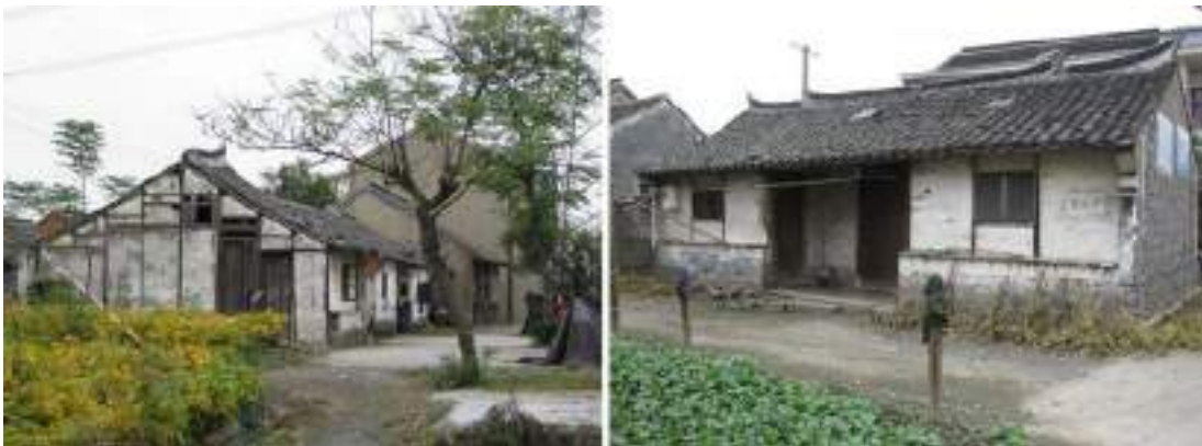
Figure 10. Dilapidated and abandoned houses in the Nankun Village.
