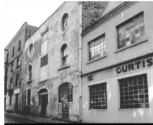
5. Comparison of facades, Temple Lane South, Dublin, 1984 © National Photographic Archive, and 2008, © Anna-Lisa Müller
