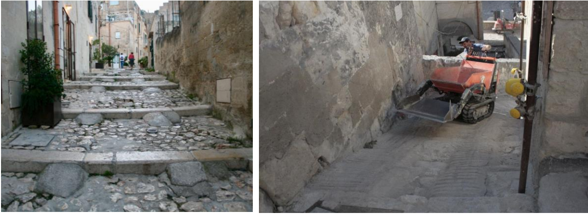
Figures 10 and 11. Adjustments on stairs for inclusive mobility, Matera, southern Italy. Personal archive.
