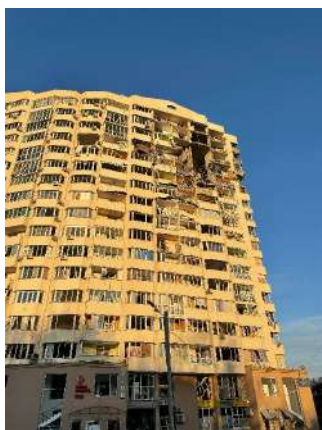
Figure 7. Destroyed house in Chernihiv (Retrieved from: https://unsplash.com/ )
