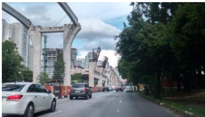
Figure 2 – Abandoned light rail works in São Paulo. Source: the author, 2016.
